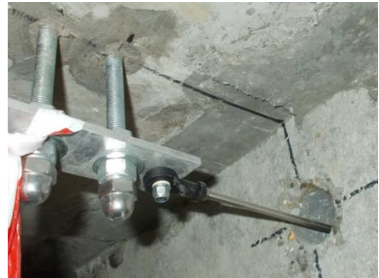
Gauges span two in-situ joints
